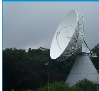
통신기기 Communication Equipment
